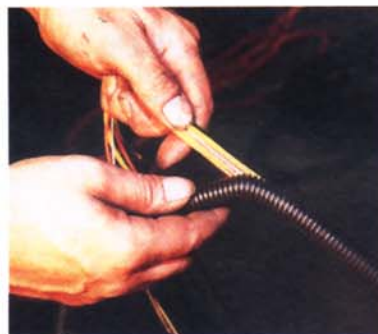
14. For a nice, neat installation, the SPAL Dual Fan electrical wire loom was encased inside some convoluted tubing.
