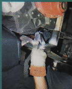
21. A&B With the engine mount squared, level and true, Brian put down some penetrating TIG-welds.
